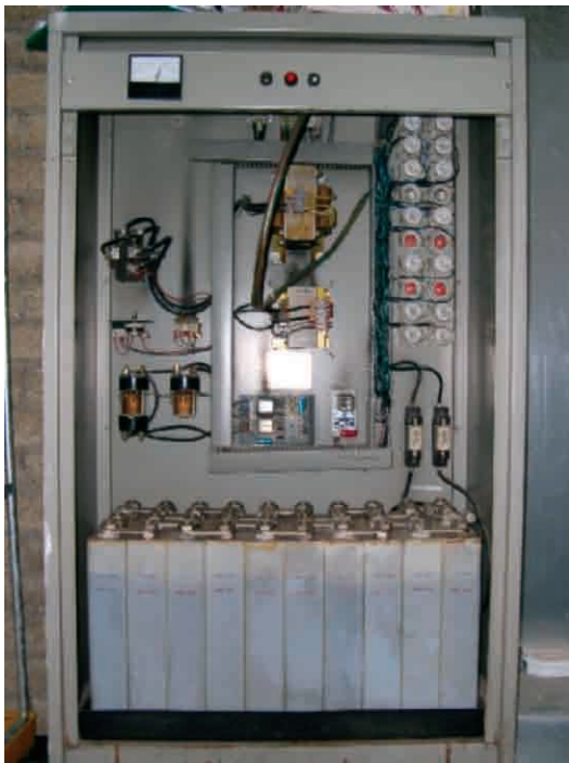
Centrale noodverlichtingunit in conditie 3
